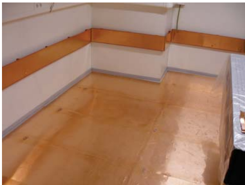
(c) Interior view during construction 2. The floor is covered with a 300 \mu\text{m} thick copper sheet.
